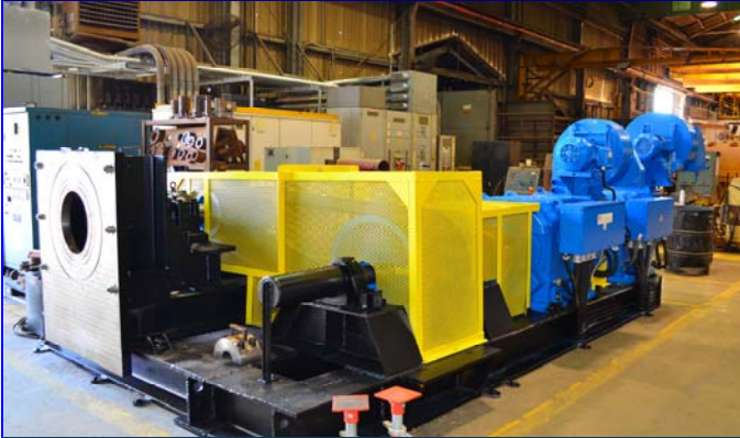
1000-kW Generator Load-Test Service
